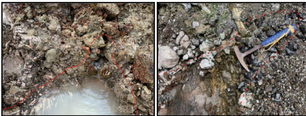
Figure 4. Seepage in Dike
