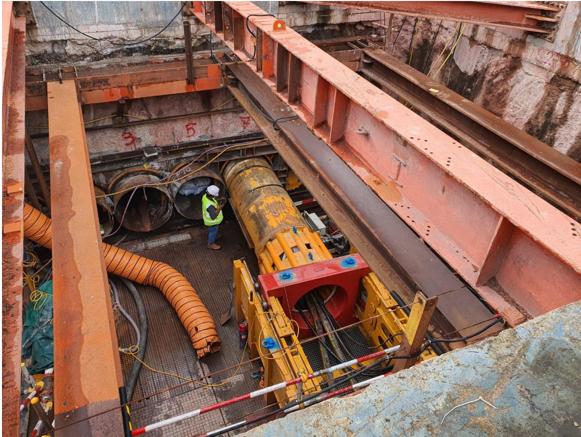
Figure 15. Photograph of micro tunnel boring machine being launched from the launching shaft (entrance).
